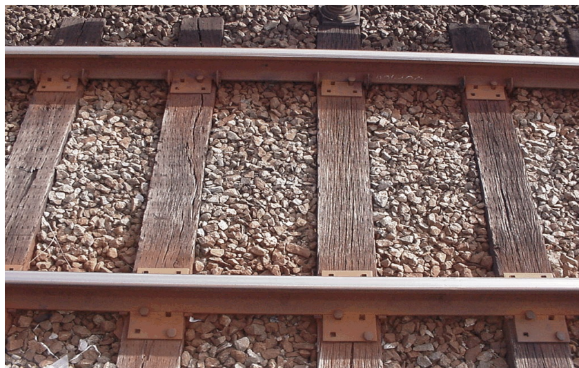
Ballasted Track, Cheverly Station
